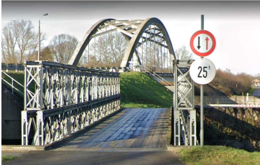
A double truss, double-storey (DD) Bailey bridge over a drainage canal in Nijlen near Antwerp. Belgium
