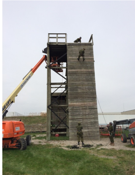
Members of 2 Combat Engineer Regiment rappel down and prepare the high wall for deconstruction.
