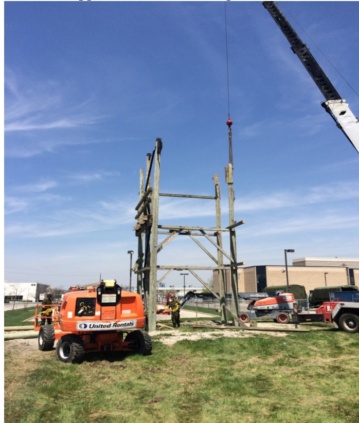
Sappers from 2 CER removing the last of the support bracing before the posts are cut and removed.
