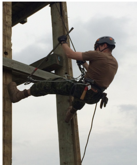
Cpl Fugere of 2 Combat Engineer Regiment works to remove the last decking board while stabilizing between two supports.
