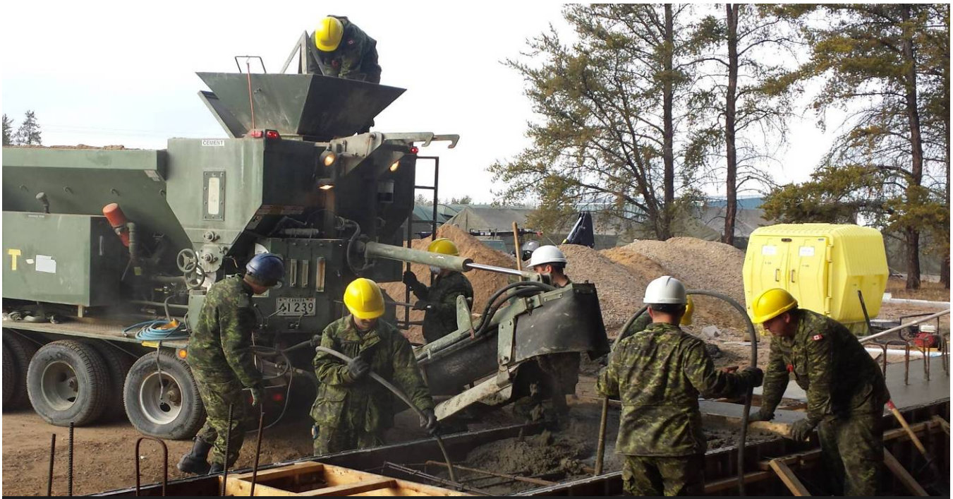
17 Wg members pouring concrete using the VCM for the front footing of a C-Span
