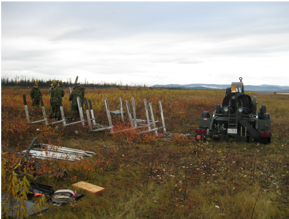
86 ASU techs install the KM stake-line used to anchor the MAAS during aircraft engagements
