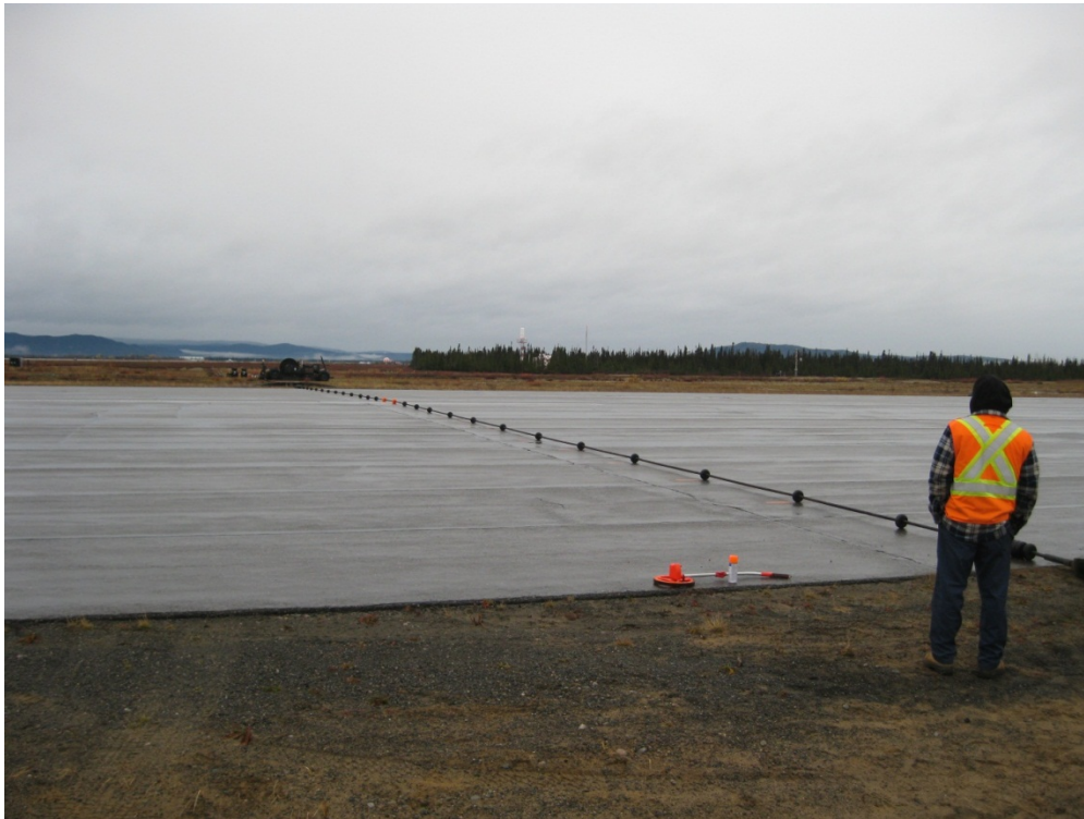
5 Wing Goose Bay SERCO contractors view the finished product and prepare for handover
