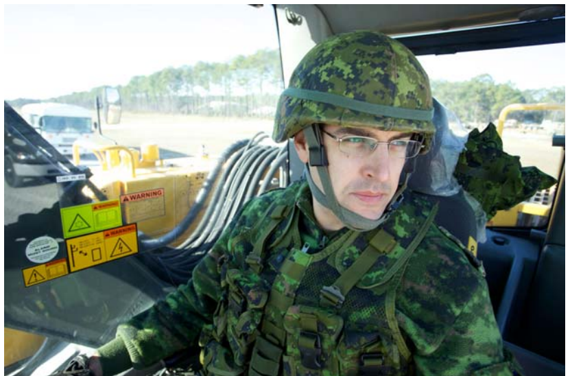
A mobile support equipment operator from 19 Wing Comox, B.C., operates an excavator to complete a runway crater repair during the airfield damage repair portion of the final exercise during the Silver Flag training exercise.
