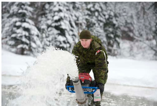
Spr Maxime Thibault floods the ice to increase the load-bearing capacity of the bridge and allow vehicles to cross. Photo: Lt Isabelle Provost
