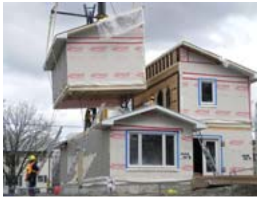
A modular home is delivered in pieces and then assembled on-site in Trenton, Ontario.
