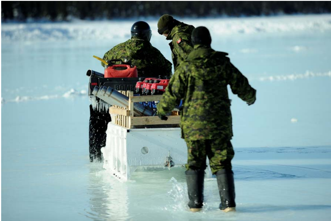
Members of 5 CER smooth out the layers of water on the ice runway.
