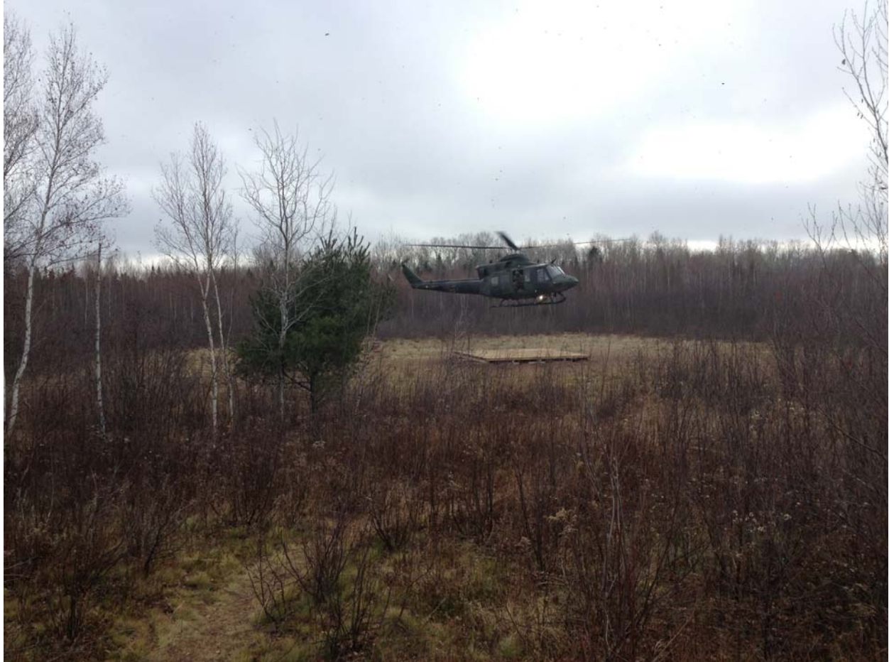
Wooden Helipad constructed by 53 Construction Troop and Construction Engineer Officer Course at AS-7. Photo by Maj Kurt Grimsrud.
