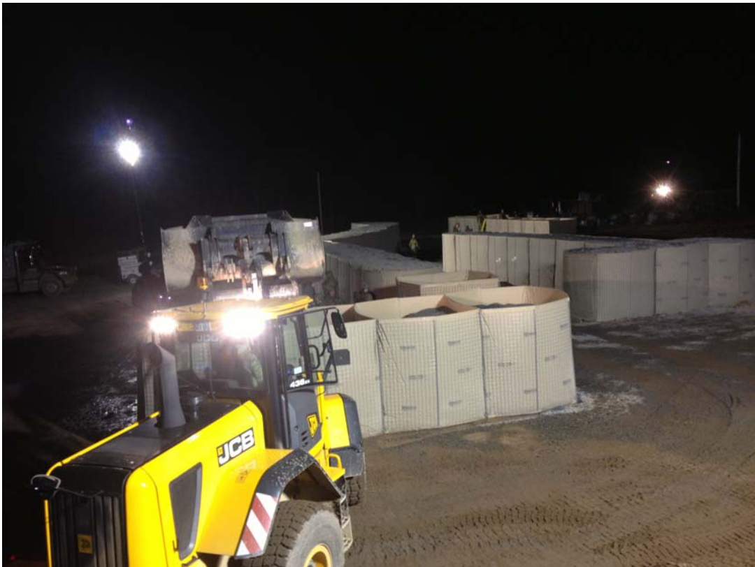
51 Heavy Equipment Troop and 53 Construction Troop with student of Construction Engineer Officer Course constructing HESCO Entry Control Point at FOB TUBOUUG (AS-6).
