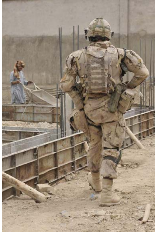
Dand District, Afghanistan; 31 July 2010 — A soldier from the Specialist Engineering Team watches Afghan labourers haul fresh concrete for the foundation of a building that will include 24 classrooms for women.
