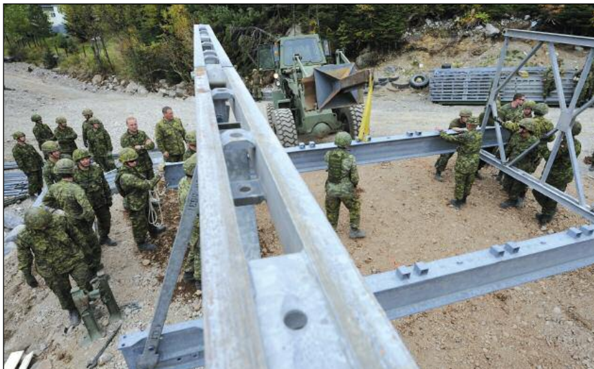
4 ESR and 56 FES sappers guide a panel into place on an ACROW® bridge to reconnect the small community of Trouty after the main bridge was destroyed by Hurricane Igor.
