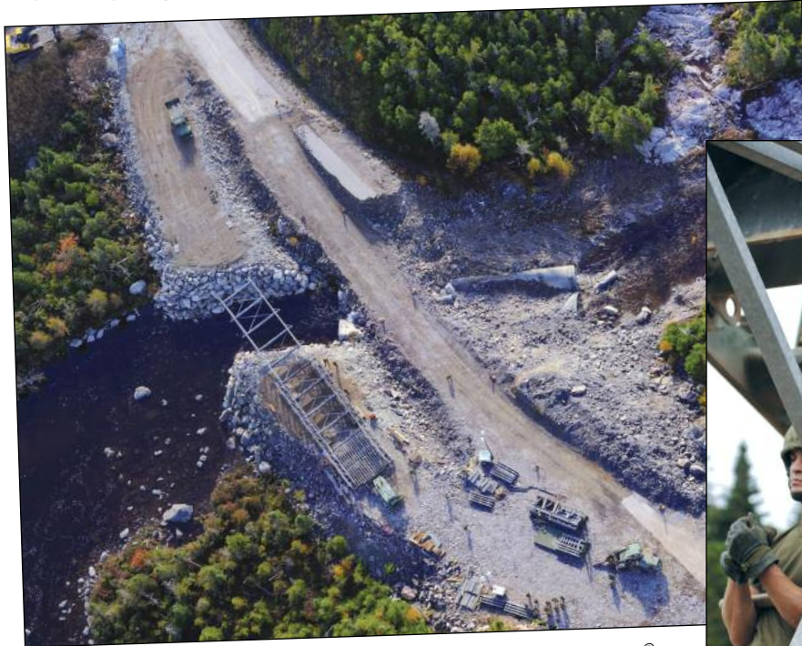
Sappers from CFB Gagetown's 4 ESR and 56 FES in St. John's, assemble an ACROW® bridge in Petite Forte, N.L.
