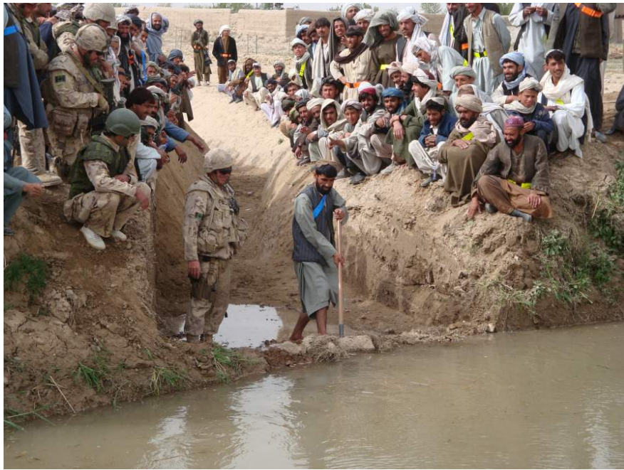
CMT 2 is implementing a newly constructed irrigation ditch in the Pashmul community of the Zahrey District, early Spring 2009
