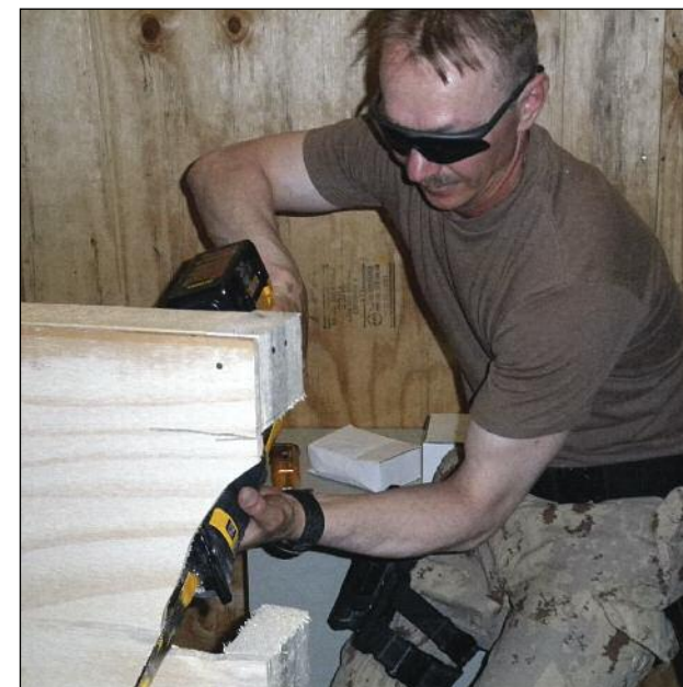
WO Bill Lynch, from 1 Engineer Support Unit based in Moncton, saws an access hole in a wall unit for the newly constructed HQ of the Canadian Contribution Training Mission – Afghanistan
