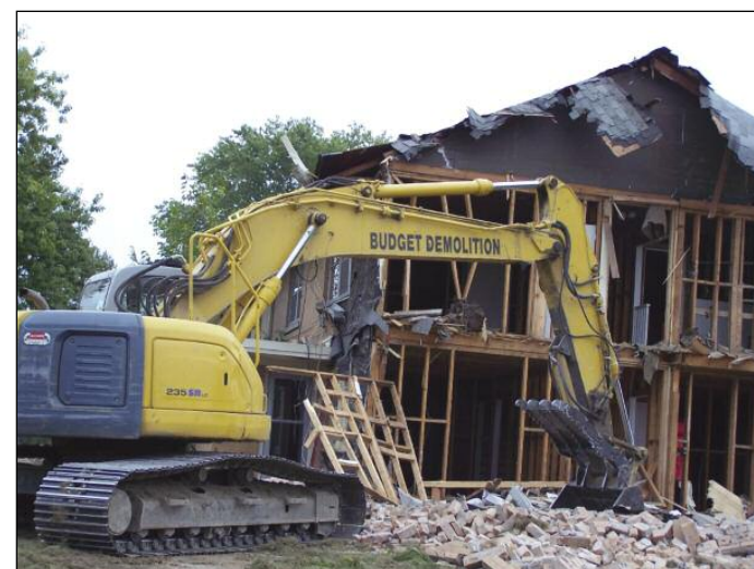
All reusable material is removed from a house under demolition, and the rest is chipped or crushed for recycling.
