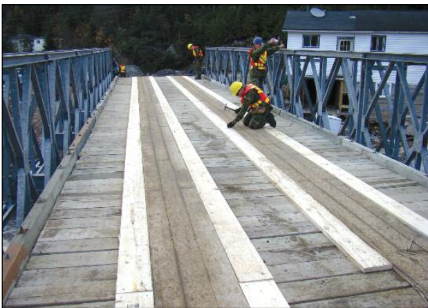
Engineers from 56 Engineer Squadron helped build a bridge in Trouty, N.L., after Hurricane Igor.
