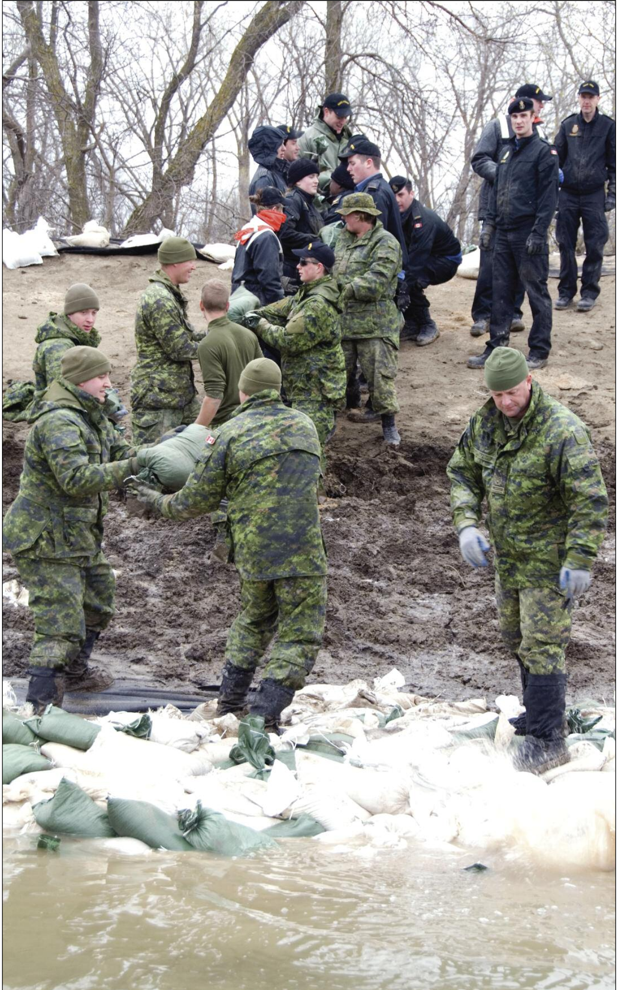
Naval reservists and 1 PPCLI soldiers work together to reinforce a dike in Manitoba.
