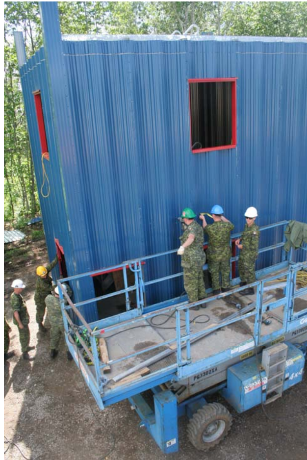
The new firefighter training tower is being built behind the Valcartier garrison Fire Hall.
