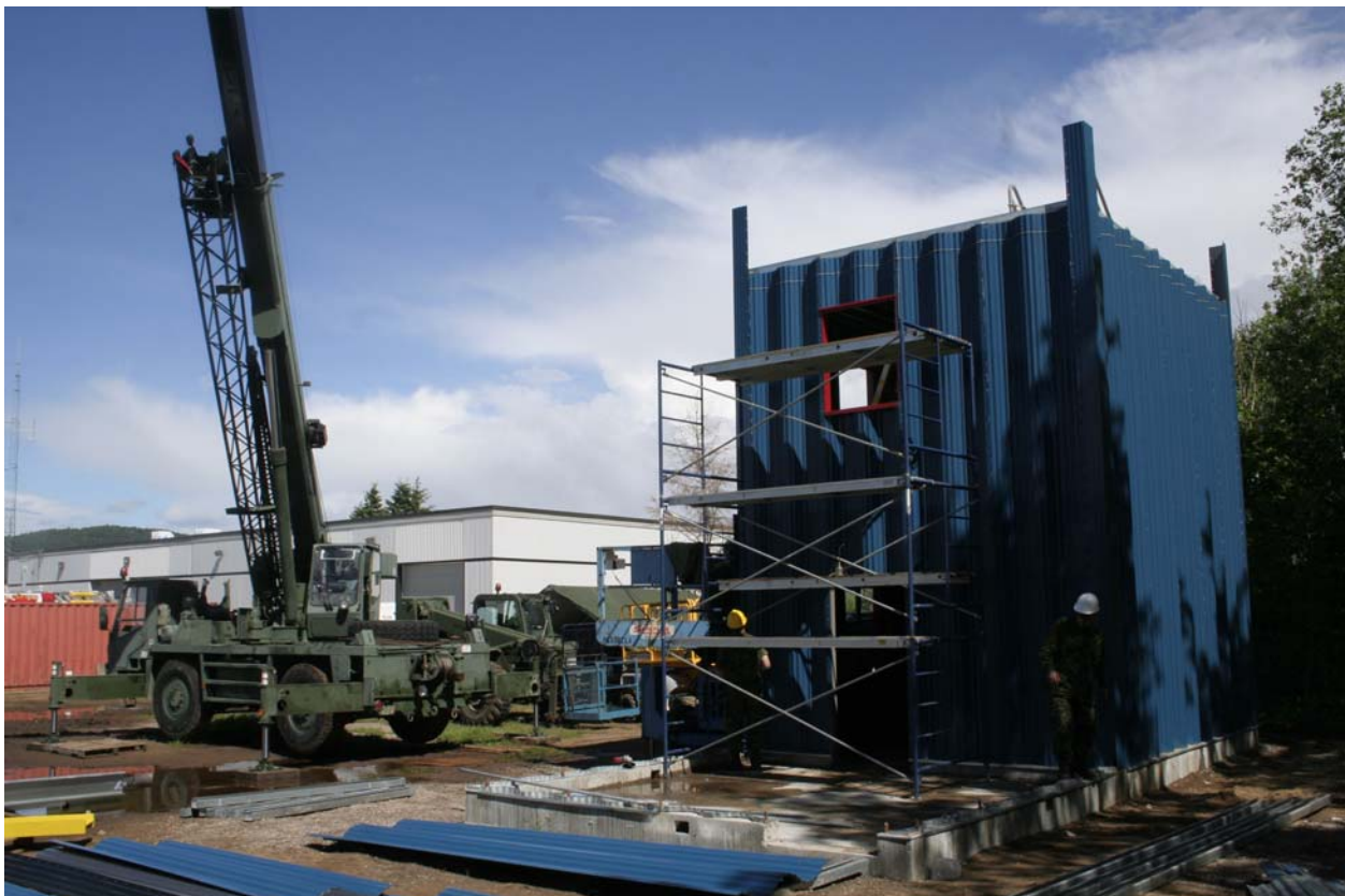
5 e Régiment du génie de combat Construction Troop and 3-10 Engineer Support Unit members are building a 4-story training tower for the Valcartier garrison firefighters behind the Fire Hall. As of 7 June, engineers had two stories built.
