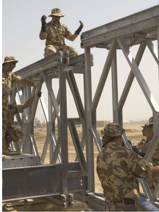
Romanian Army field engineers assemble a steel bridge during a training session.
