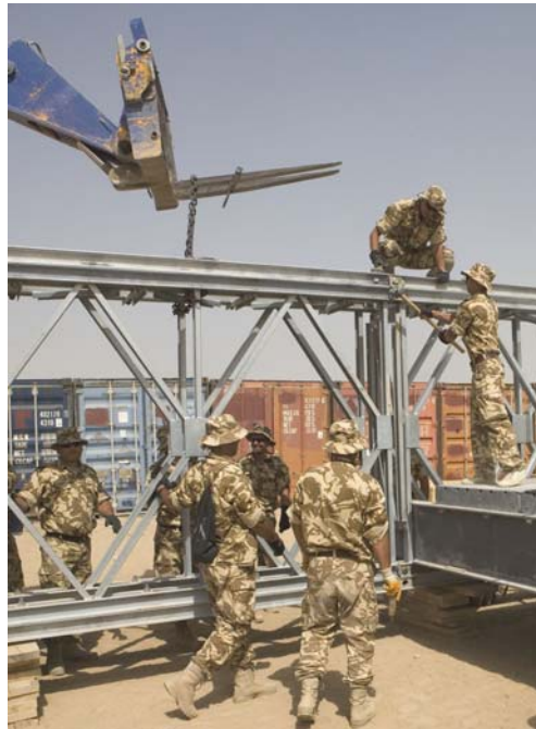
Romanian Army field engineers in training use a forklift to join bridge sections.
